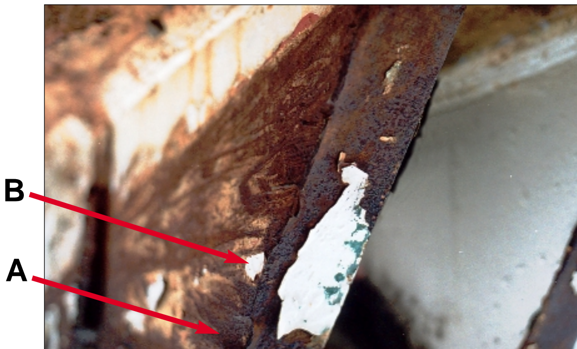
FG 13. The port hydraulic lug. Note the plastic deformation shown by arrow A made in the direction of the arrow, and the sharp edge shown by arrow B. Note also that there is paint on the very edge of the lug also shown by arrow B. (This picture can be compared with the German Expert Group picture E9 on the next page, where the complete lug is shown.)
